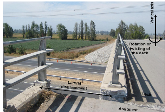
Fig. 1. Typical damage of overcrossings after the Chile earthquake of February 27, 2010. Source: Taken from [5].
